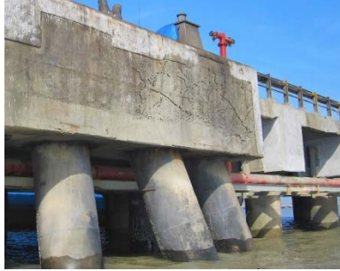
Delamination from reinforcement corrosion.
