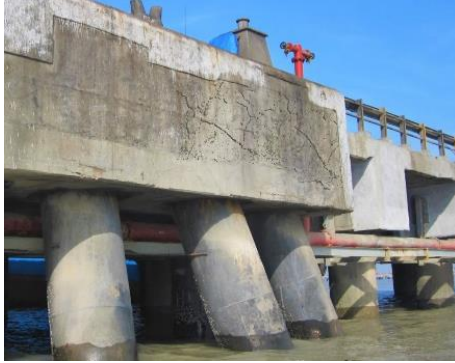
Delamination from reinforcement corrosion.
